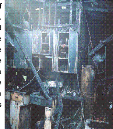
An explosion in a meth lab caused the fire that destroyed this home in Fort Smith.
